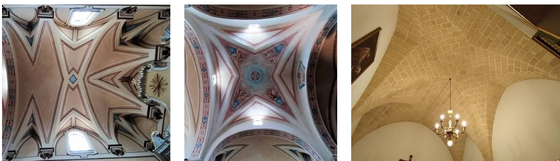
Figure 2: Vaulted ceilings: a) on the apse; b) on the transept; c) masonry arrangement (in the sacristy).
